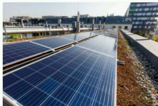
Collective PV system at Lavaterstraße
