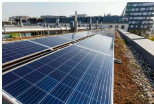
Collective PV system at Lavaterstraße
