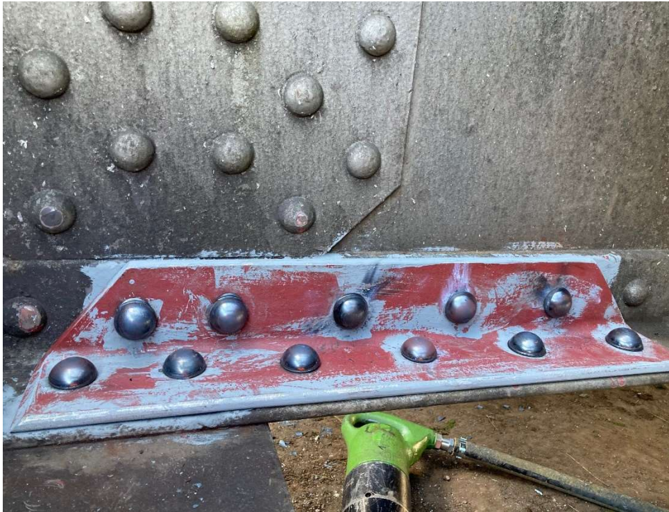
Fig. 27: Example of strengthening by adding component using a riveting device (Foto: F.Looser).
